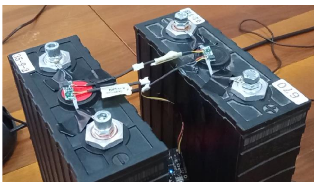
Figure 11: CMU mounted on daisy-chained LiFePO 4 prismatic batteries.
